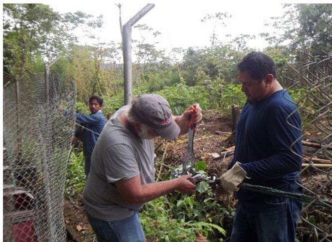
Darrell working with Vinicio and other maintenance helpers fixing a fence that was damaged by falling trees during a jungle storm a few months ago.
